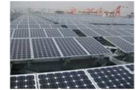
Roof-top Solar Power Systems
