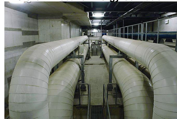
Heat Supply Pipe for District Heating and Cooling
